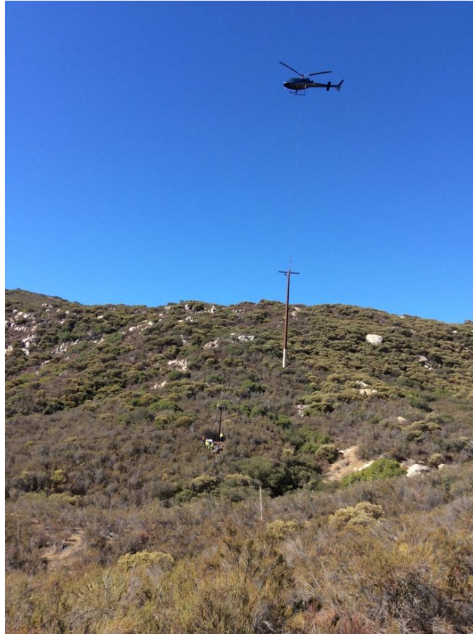
Photo 2: A crew was observed utilizing helicopter external load operations to set the pole at P278714 (C157).
