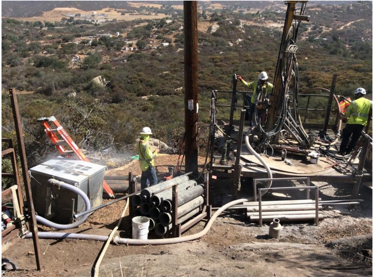
Photo 4: A covered containment box was used to trap drill cuttings and reduce dust emissions during micropile drilling at Z571420 (TL 6957), in accordance with APM AIR-05.
